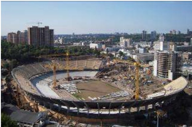
▲ Work is continuing around the clock on refurbishing the National Olympic Stadium in Kyiv, the proposed venue for the final of UEFA EURO 2012.
